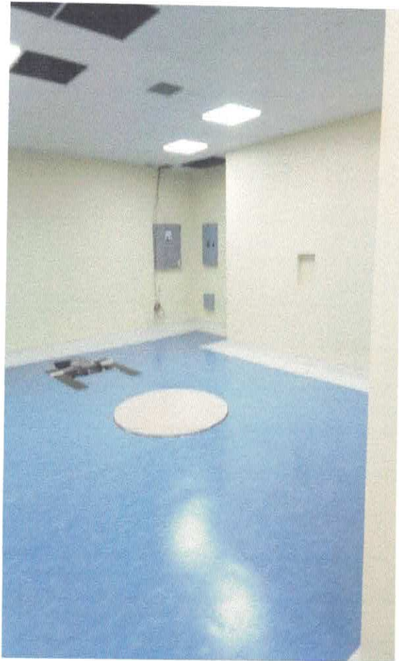
Interior of Linear accelerator Bunker and Control Room
