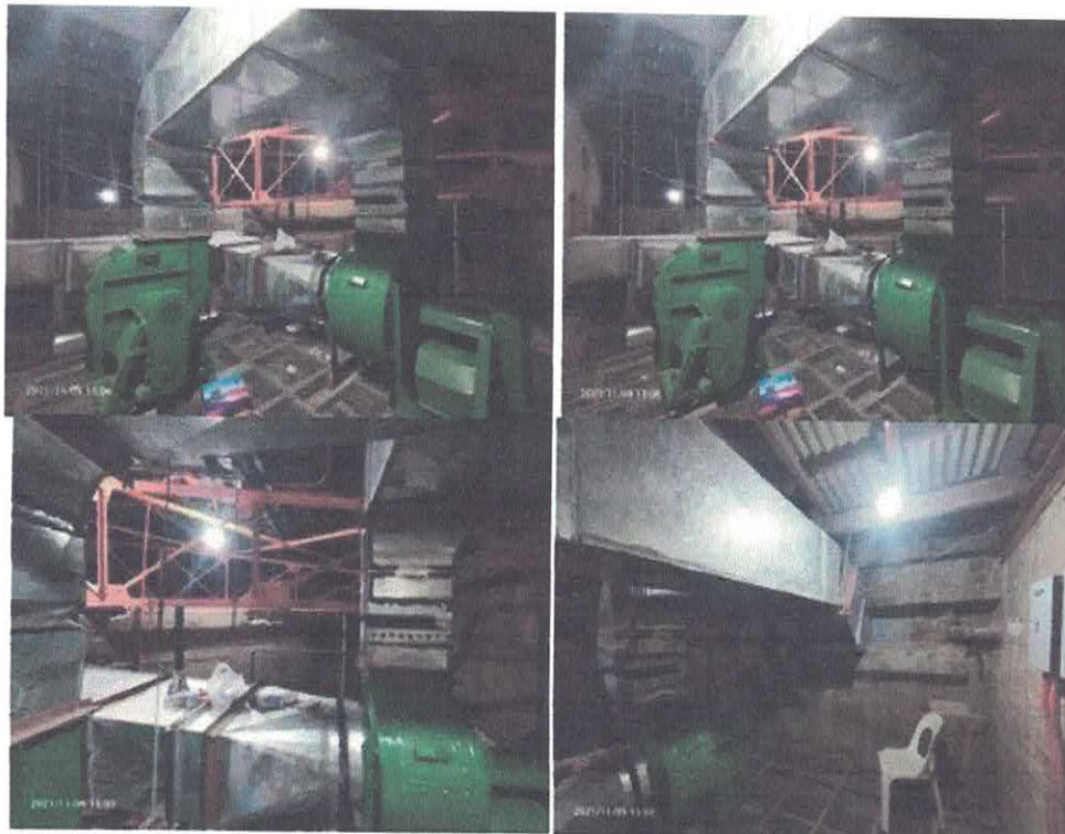
Ducts, Exhaust Fan & Damper
