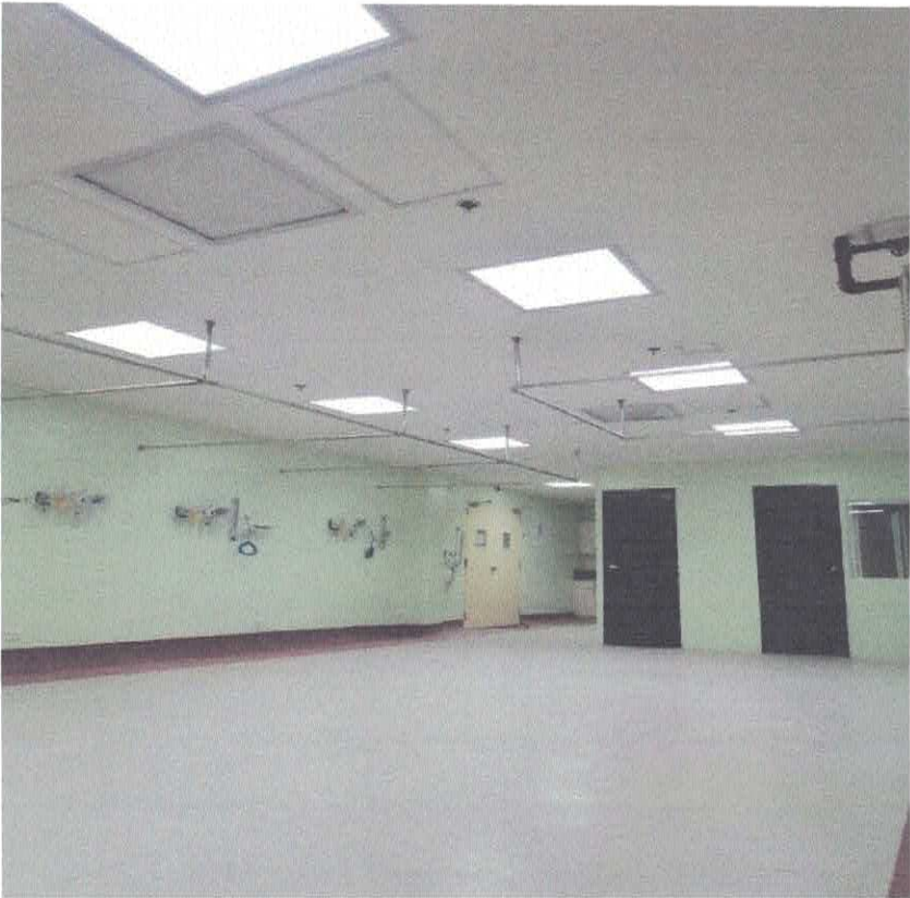
MICU ISOLATION ROOM
