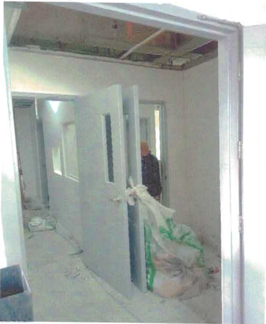
Ante Room 1 (Going to Specimen Receiving Room; & Sample Prep Room)
