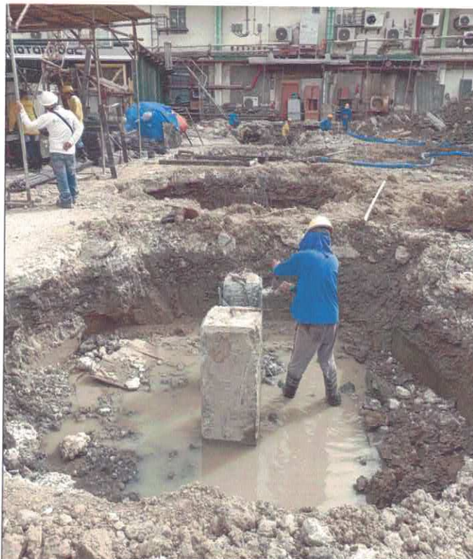
Project: Alteration of Radiotherapy Building to Include a New Linear Accelerator Bunker and Renovation of Various Area
